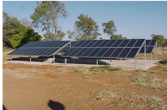
Figure 6 BP3160 Solar Array
